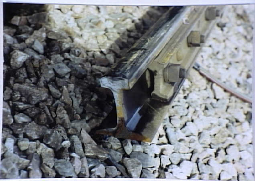
Photo 4. End view of the East end rail segment at the POD and the internal rail defect that measured 24 1/2 inches from the East end bolted rail joint
