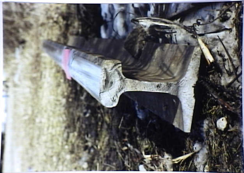
Photo 6. End View of the second internal defect that measured 98 1/2 inches from the East end bolted rail
