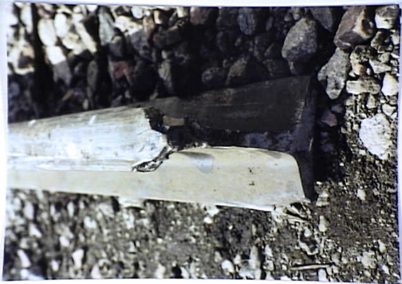
Photo 8. End view of the matching rail face for the second internal defect that measured 98 1/2 inches from the East end bolted rail joint
